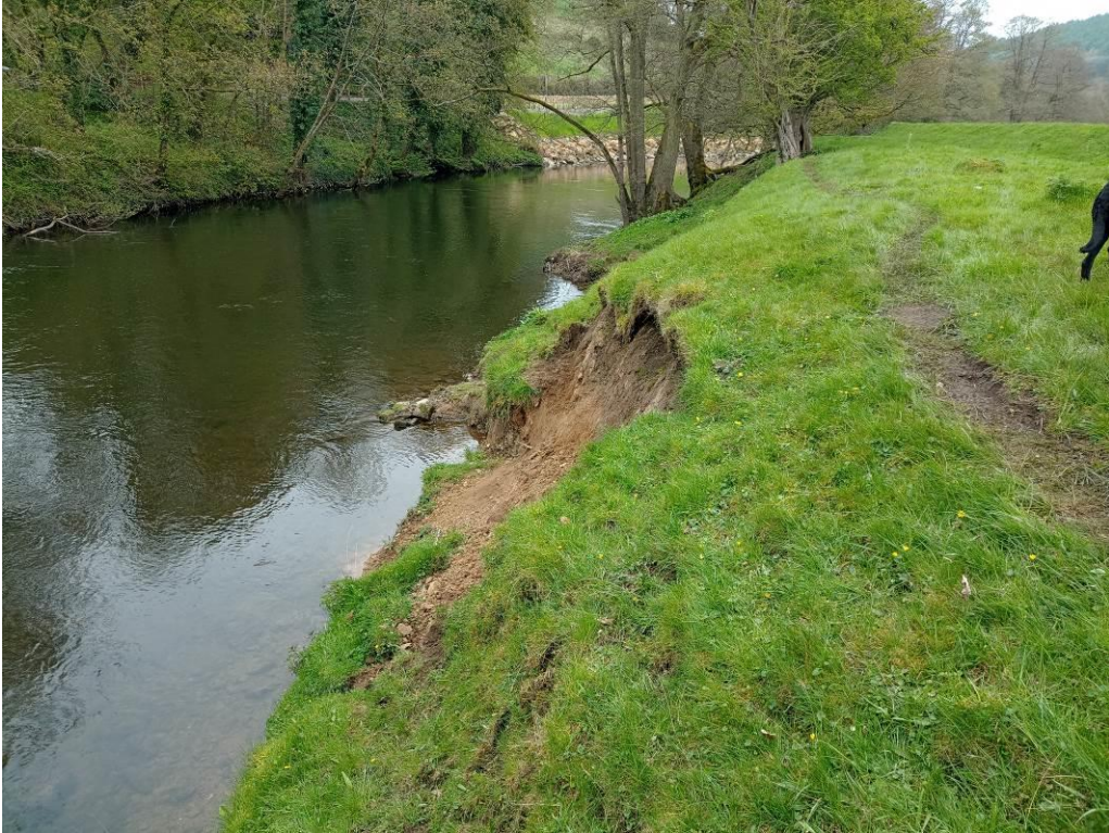
Photo 6 Possible site of a fallen tree, illustrating shallow root horizon of grass and reduced bank stability.
