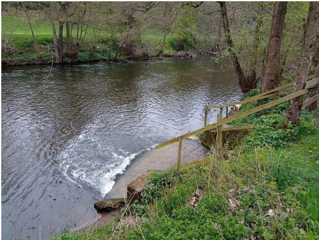
Photo 8 Treated effluent discharge from Matlock sewage treatment works.
